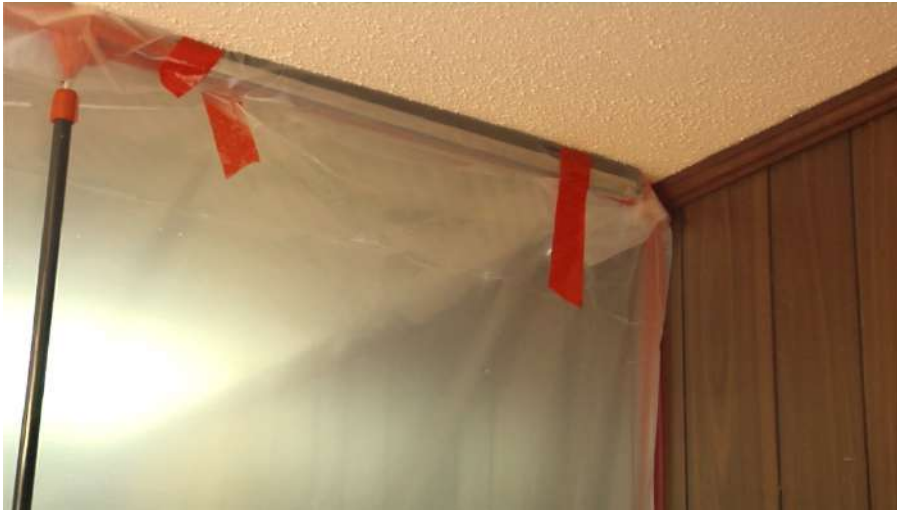
1. Isolation barrier installed to divide a room with asbestos popcorn ceiling into two distinct test areas
