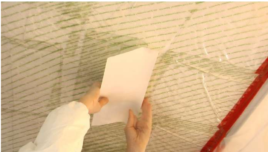
2. MoldHold sheets were applied to one side to minimize possible asbestos exposure
